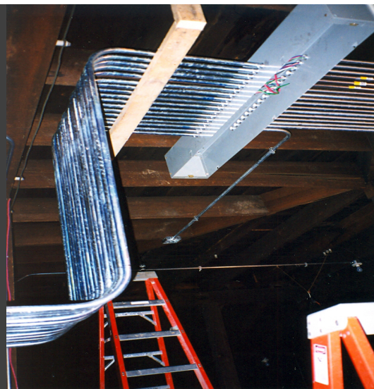
Electrical system - after
