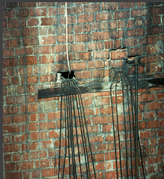
Electrical system - before
